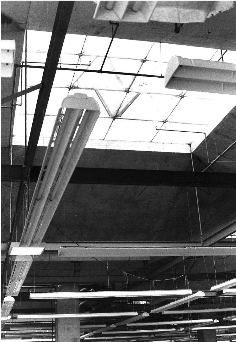
Figure 12. One of the skylights seen from the inside of the factory, Harrisburg (PA), 1970. (Fondazione Renzo Piano)
